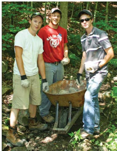
▲ MNR crew, Brad Immerseel, Lindsay Brown and Andrew Meiklejohn placing rocks on the stream bed.
